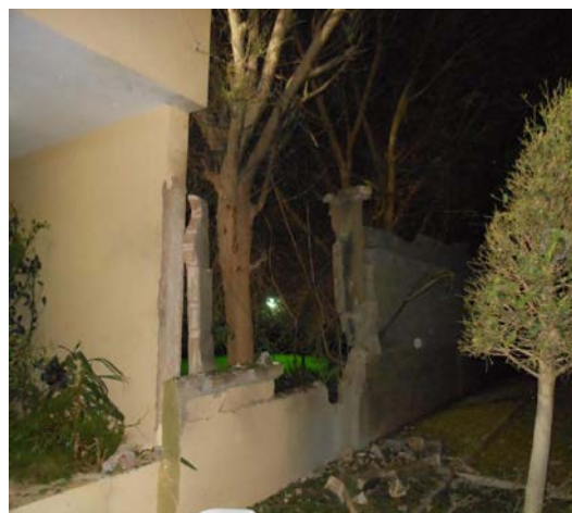
Damaged wall at consulate compound, House Committee on Oversight and Government Reform, 2012
