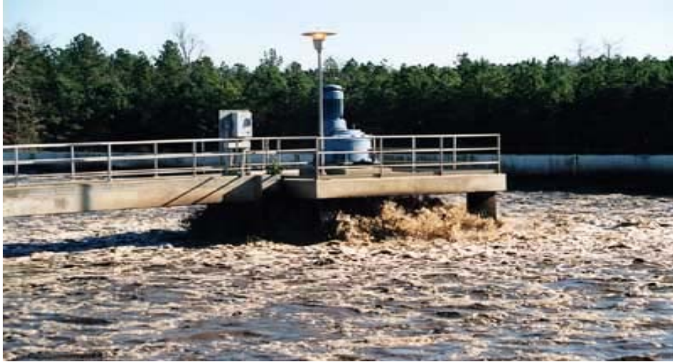
Figure 7 Wastewater Aeration Basin
