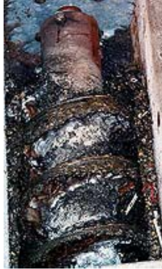
Figure 5 Grinding Large Particles in Wastewater Prior to Removal
