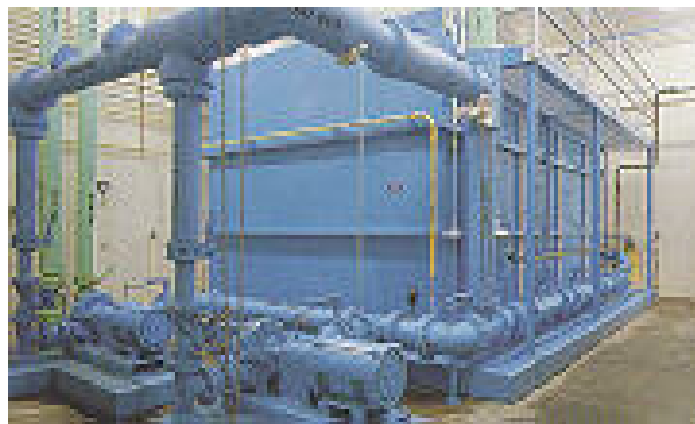
Figure 10 Wastewater Filtration Unit
