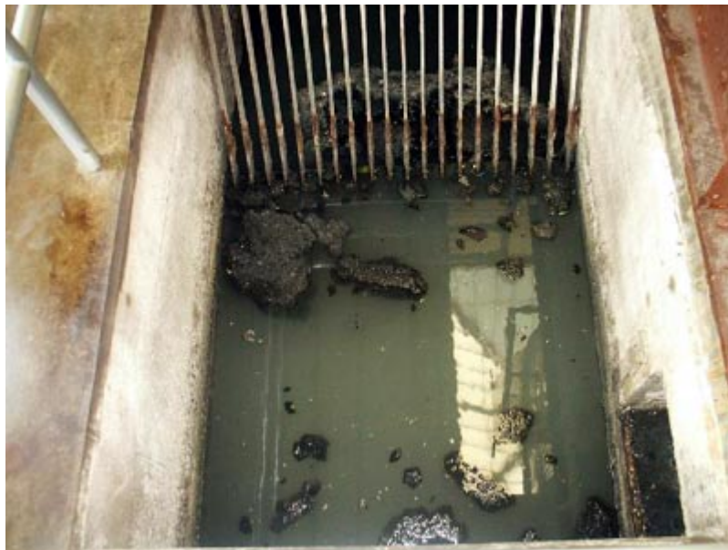
Figure 4 Wastewater Sewer Screen
