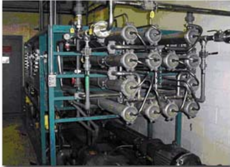
Figure 11 Small Reverse Osmosis Unit for Tertiary Wastewater Treatment
