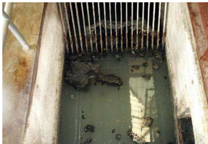
Figure 3 Wastewater Sewer Screen
