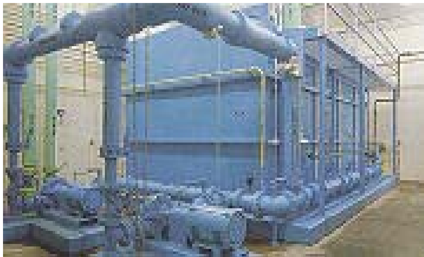
Figure 9 Wastewater Filtration Unit
