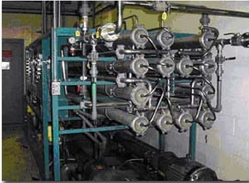
Figure 10 Small Reverse Osmosis Unit for Tertiary Treatment of Wastewater
