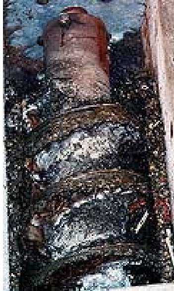
Figure 4 Grinding Large Particles in Wastewater Prior to Removal
