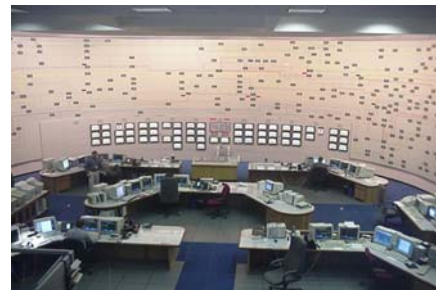
Figure 19 SCADA System Control Room
