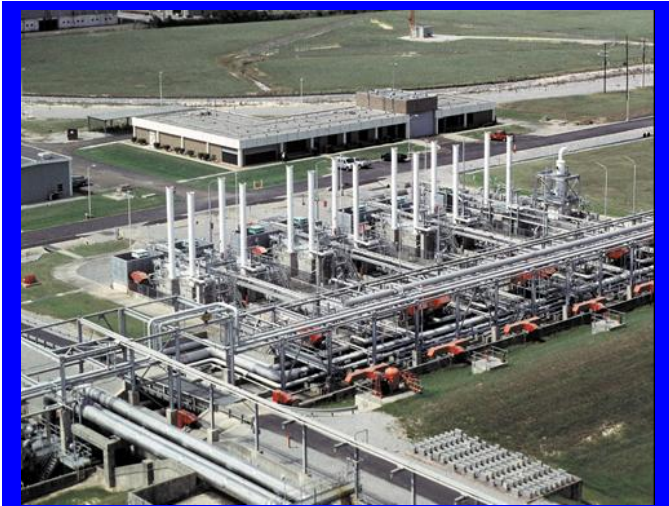
Figure 2 Water Bath Vaporizers
