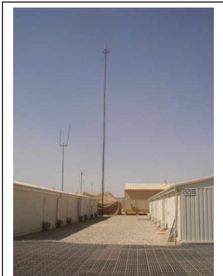
Figure 6: PTM-100 80 foot antennae significantly increased the range of RIAB transmissions.
